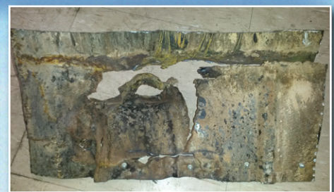
The damaged section of floor cut out.
