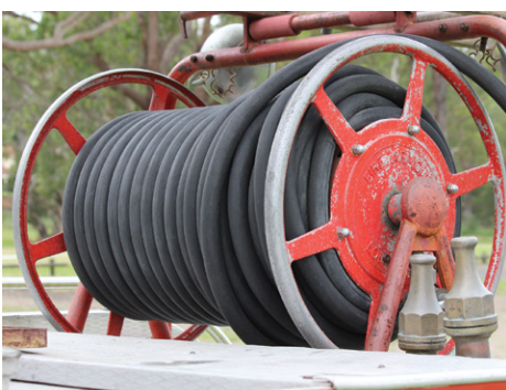
Hose reel for first response work only.
