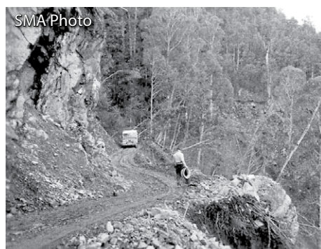
By 1953 many roads were in the process of being widened for heavy vehicles.
